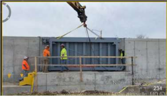
Caruthersville, MO Floodwall (BBA18)
